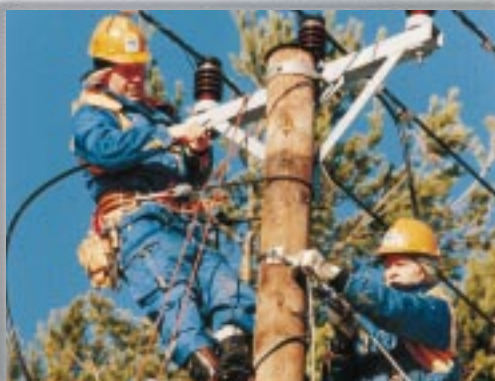
Hans Löwegren and Calle Ersson work on a new 10 kV power line on the island of Ornö off Stockholm.
