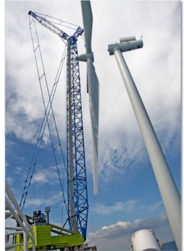
Lilgrunden Wind Power Plant, 2007-08-04 Installation of a wind turbine from M/S See Power.
